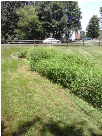
Riser structure, obscured by vegetation
