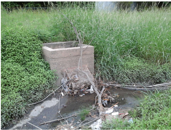
Riser of dry pond showing blocked screen
