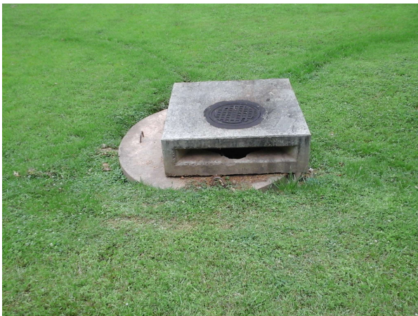
Outlet of stormwater pond out of alignment.
