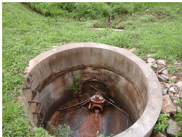
Riser interior with flow constrictor valve
