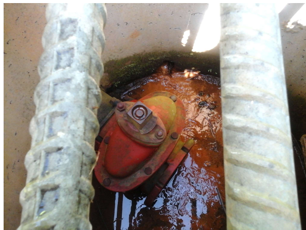
Interior of high flow outlet showing restrictor valve
