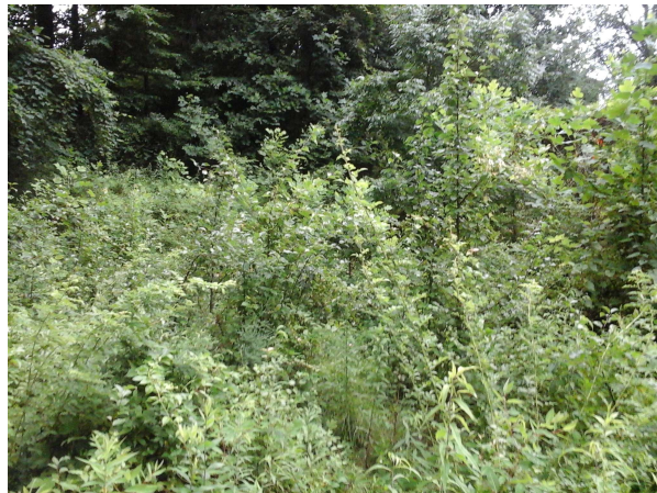
View of overgrown vegetation in dry pond facility
