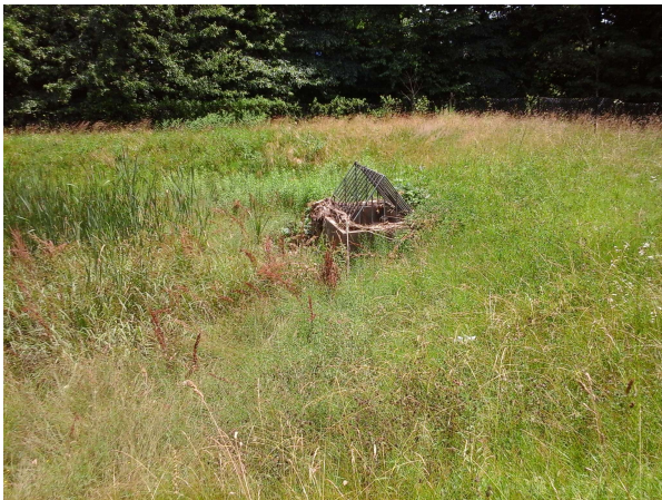
View of dry pond riser
