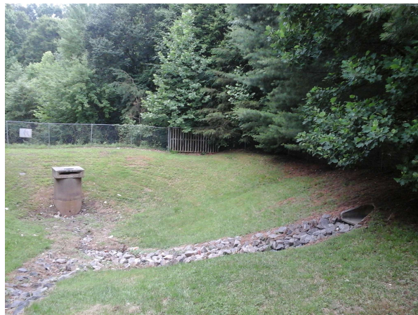
Dry pond showing channel configuration and route to riser
