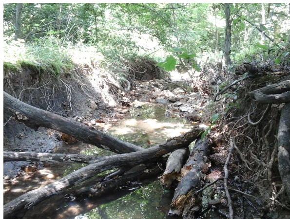
View of erosion damaged ephemeral channel downstream of culvert
