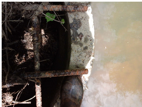
Top view of high flow riser, showing backed up water
