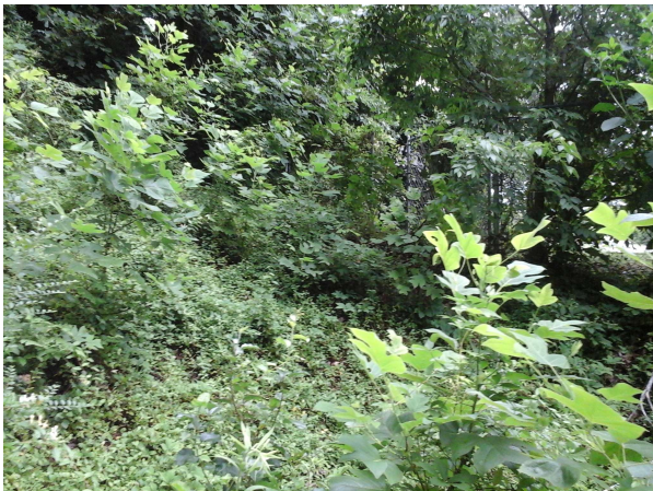
View of overgrown vegetation and small trees in dry pond facility
