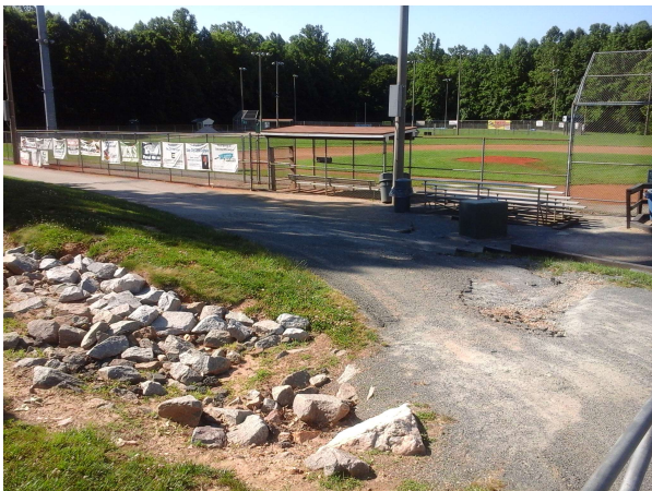
Area east of stormwater pond showing erosion due to flow bypassing blocked culvert
