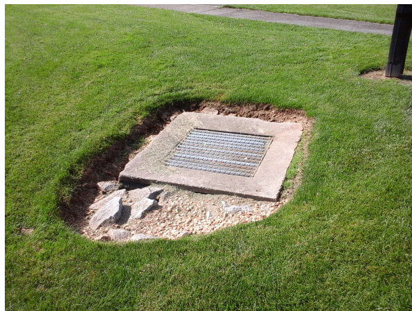
Yard inlet to east of driveway showing localized erosion
