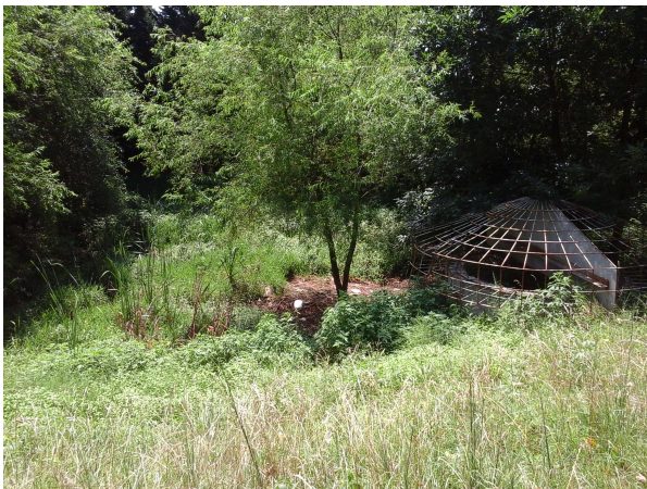
View of dry pond riser
