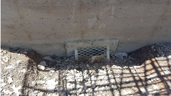
Partially blocked low flow orifice
