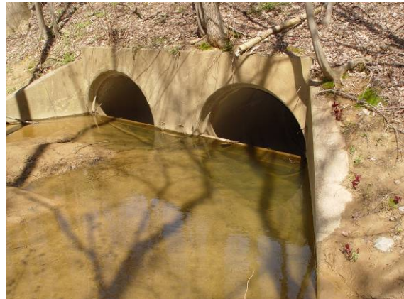
FIG 22: Culvert Retrofit that Reduces Discharge Capacity, and does not accommodate sediment and animal passage.
