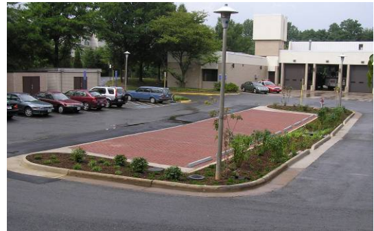
FIG 17: Northern Virginia Retrofit Using Porous Pavers and Conversion of a Parking Island to a Bio-Infiltration Facility
