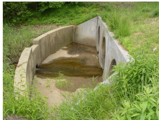
FIG 21: This Dry Pond Structure was Built in Conjunction with the Roadway Culverts on a Small Drainageway
